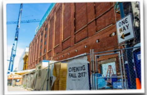
Above: The Museum of the Bible is under construction and scheduled to open in the Fall of 2017. Find out more at museumofthebible.org
